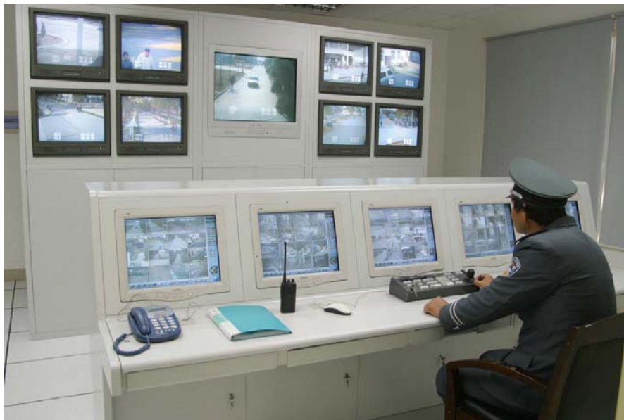
Figure 1. Remote monitoring system of operation room
