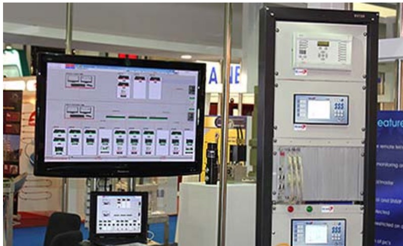
Figure 5. Electrical automation control equipment
