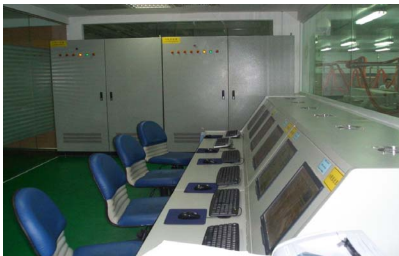
Figure 6. Electrical automation control equipment (b)
