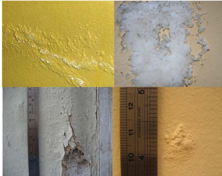
Figure 7. Common defects in painted interior walls: swelling, efflorescence, cracking and blistering
